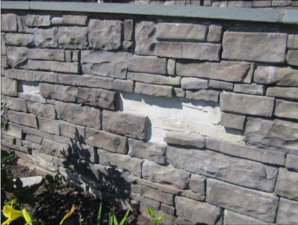
Retaining Wall - Missing Stone Veneer
